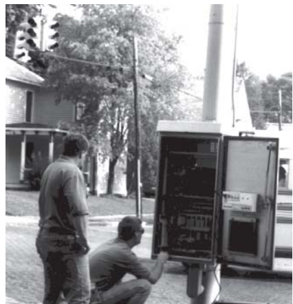
Photo 2 Field testing of cabinet primary surge suppressor with a dark intersection. An extra person was needed to direct traffic during the time of no indications.
